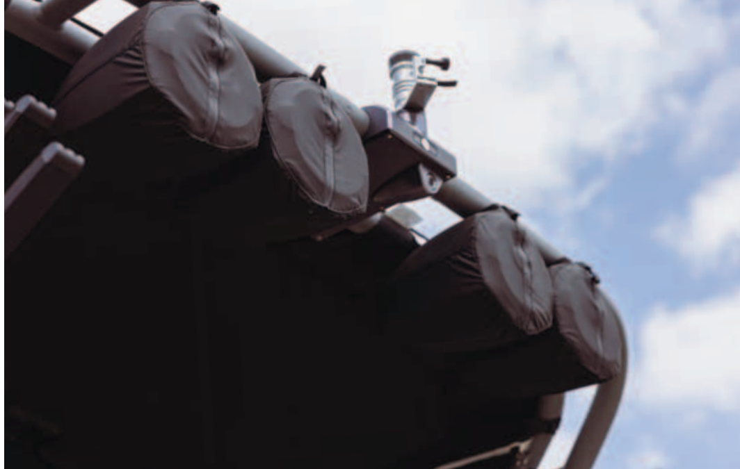
Installed Speaker Can Covers
