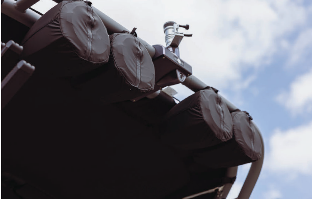
Installed Speaker Can Covers
