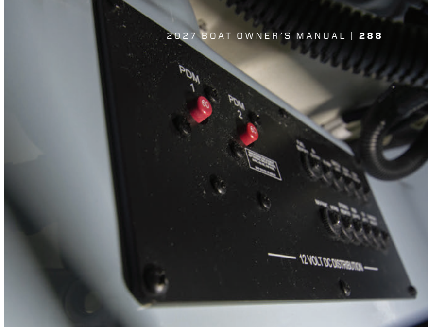
Main circuit breaker panel under the dash on the XT23
