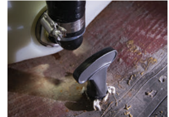
View beneath deck of properly installed center drain plug
