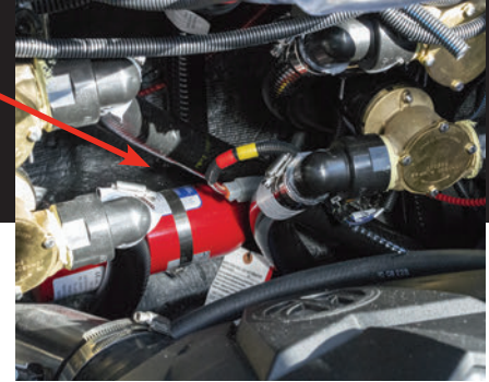
Location of Engine Fire Extinguisher
